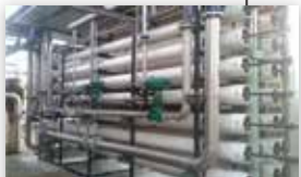
Industrial Wastewater Reuse: 6,000m 3 /d
