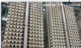
Seawater Desalination: 600,000m 3 /d
